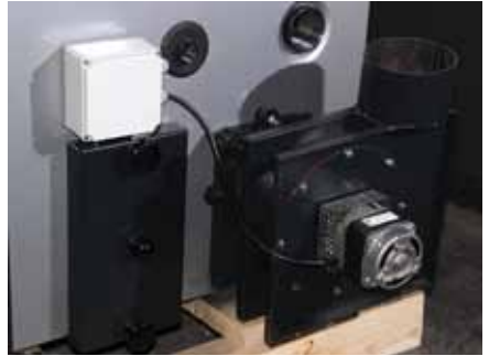
Flue gas blower installed on a fitting part.
