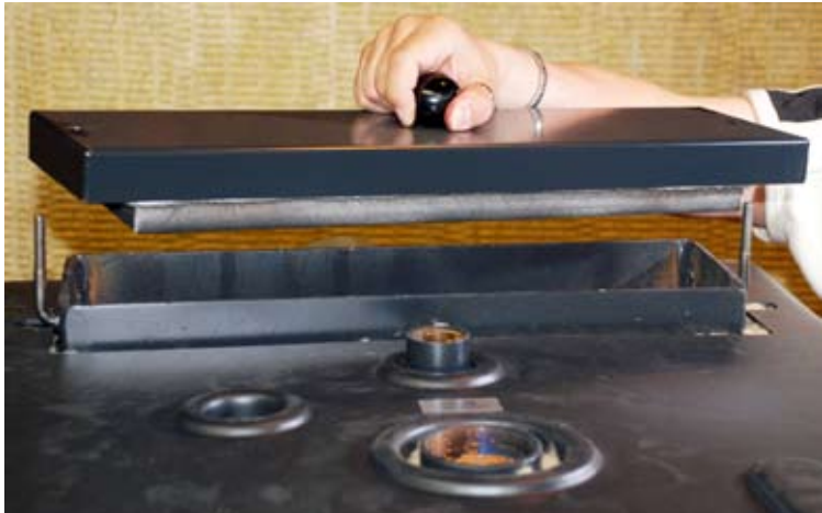
Cleaning the convectional flues. Lift the sweeping hatch at the top of the boiler and clean the flues with brush. Cleaning is needed few times a year.
